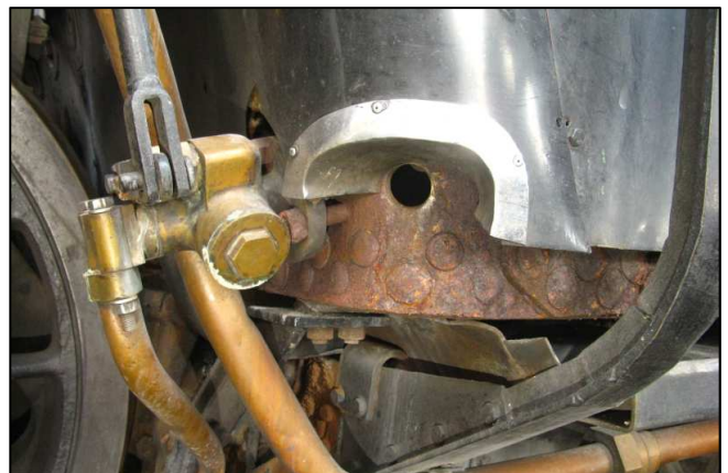
P04 - Several of 15F 3046's washout plugs had been removed as well to allow a gentle, healthy drying draft in the boiler's water space through December.
