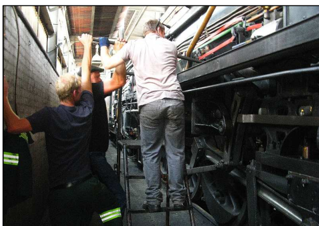
P07 - Work needed to be done on the left side die block. So the radius rods had to be manually shifted upwards to allow for access. This is how you 'change gears' on a stationary cold steam locomotive, and you have to disconnect the locking cylinder of the power reverser first.
