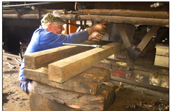
P05 - Aidan tackles the unbolting of the 21-inch brake vacuum pan for later removal. It was booked for a full strip down and inspection (And to be marked by a date when done), and new seals & roller ring as a matter of course.
