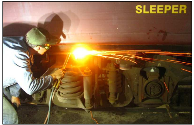
P03 - Over the years, we have removed obsolete and untidy steam heating equipment, battery bays, wiring, old pumps, axle-driven pulleys, etc. It opens up the lower coach body for access, and for addition of a train-lengthed water mains and also saves weight. (Over 8 tons on a full length tour train.) Dawie Viljoen is seen cutting away a now-unused hangar bracket for a steam heating pipe.
